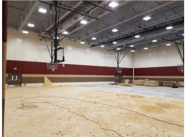
Gym painting and lighting complete, equipment installed, and sub flooring going in as of 9/15/17
