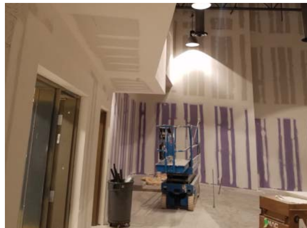
Approximately 90-95% of the auditorium has been fully mudded and sanded. Lights installed as of 9/15/17
