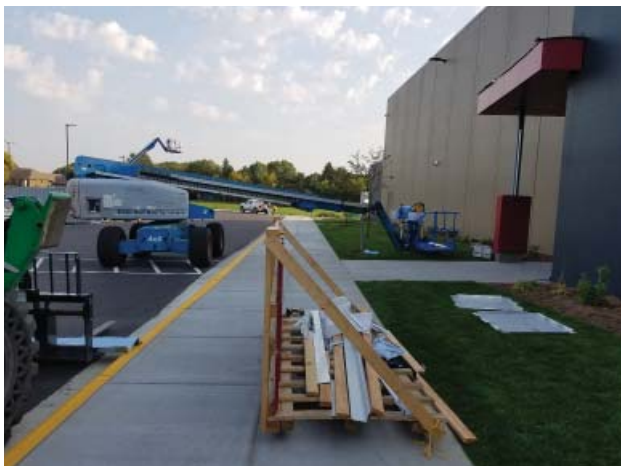
Metal panel installation (after school hours) at the east entrance as of 9/15/17
